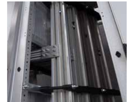
Vertical and horizontal busbar systems
