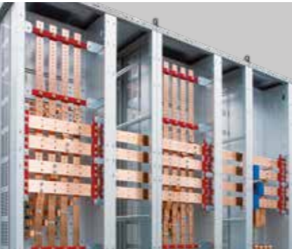
Cabinet - rear busbars: cabinet with sections and segregation form 3b. Vertical and horizontal busbar system placed at the back.
