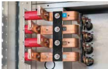
extension of horizontal or vertical circuit breakers terminals: Copper
