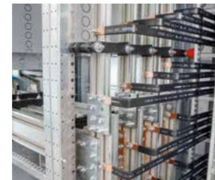
Vertical and horizontal busbar system: Vertical and horizontal busbar system placed at the back
