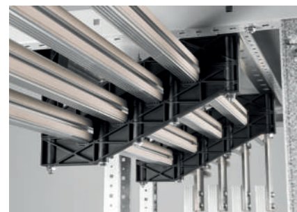
Upper area inclined busbar holder
